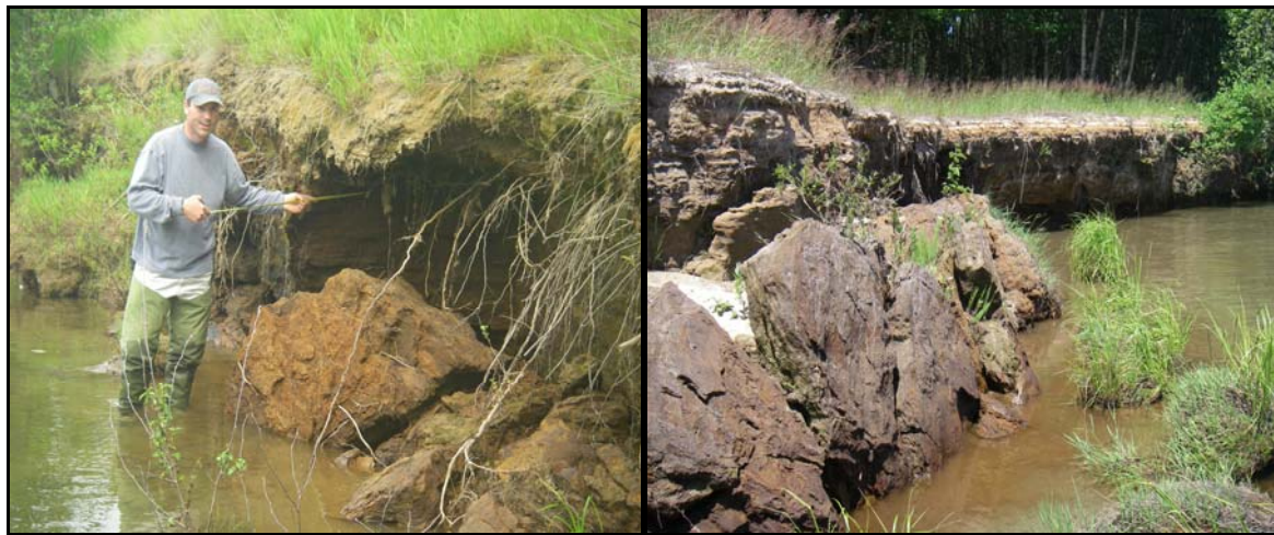
Figure 31. Undercutting and severe slumping of banks on the Lower Coeur d'Alene River.
